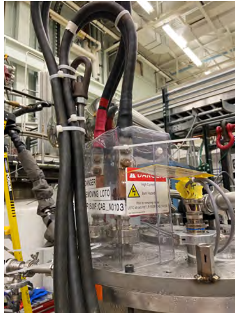
Figure 5.22 500 A power supply DC cable connection to the leads connection lugs of the coil testing assembly.
